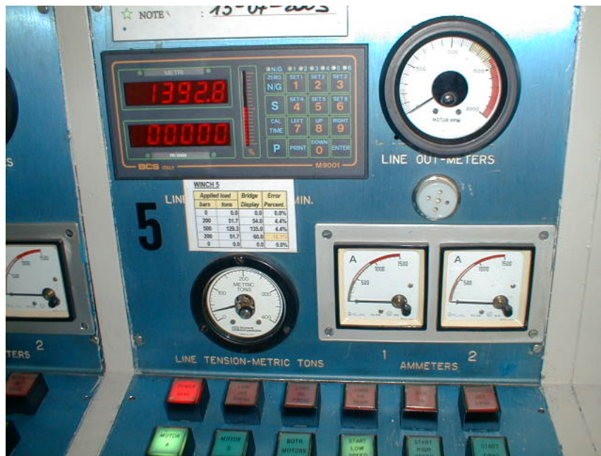
Tension meter on the winch panel
