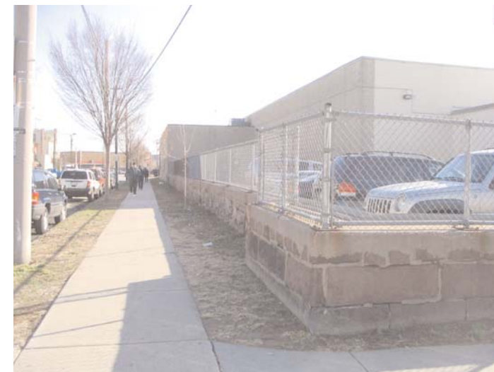
Existing Moyamensing Prison ruins (Recommendation: replace chain-link fence and repoint masonry)
