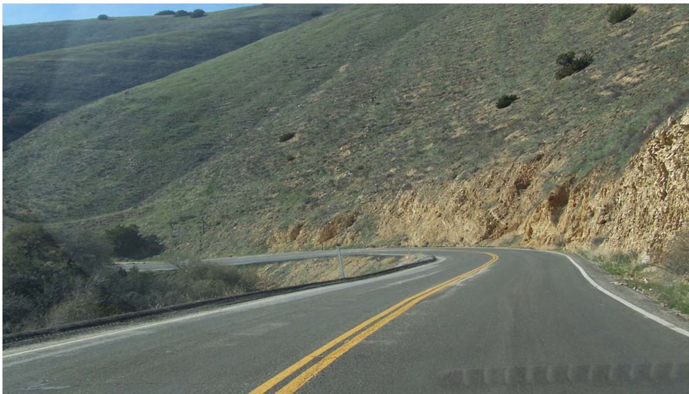
Note sharp curve and no shoulders.
