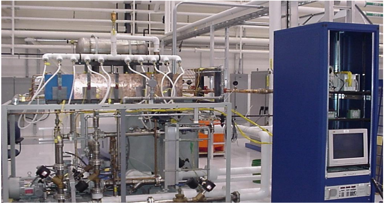
Figure 3. FCtec thermal load bank test stand.
