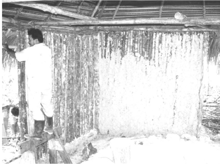
Figure 2.8 Construction of a traditional bajareque structure at El Pilar. The walls are being plastered with a mixture of sascab, grass, and water.
