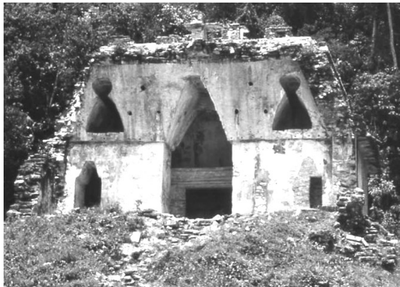
Figure 5.13 Holes in the vault mass of the Temple of the Foliated Cross, Palenque, Chiapas.
