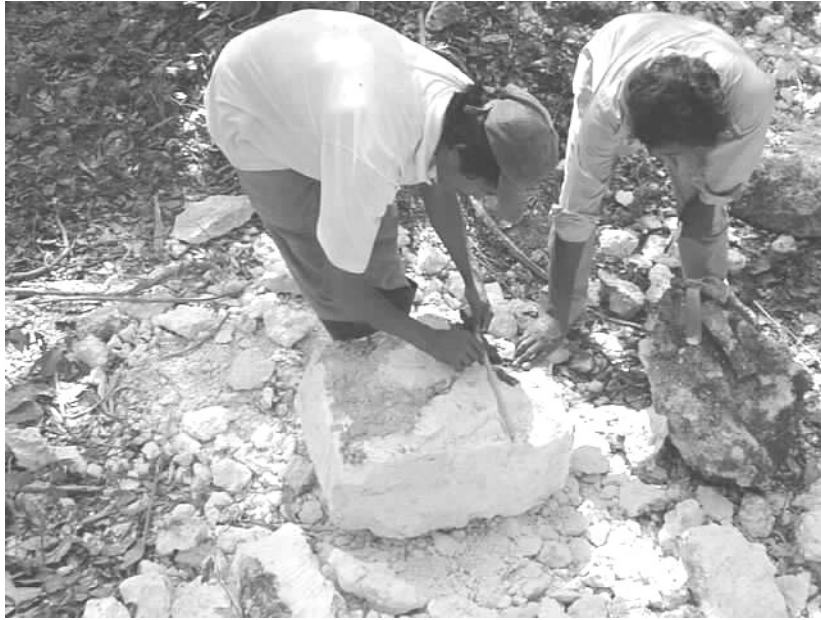
Figure 2.3 Workers at El Pilar trimming limestone blocks for consolidation work. Note the hatchet they use (on top of block to the right).
