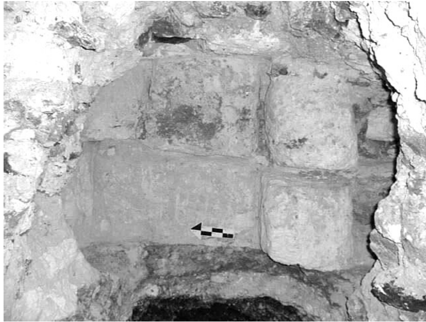
Figure 3.10 The backside of the megalithic retaining wall underneath structure EP7 at El Pilar. Note the header and stretcher bond.
