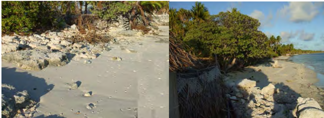
Fig. 2l: Damaged seawall (photo by Temakei Tebano) Fig. 2m: A reclaimed land
