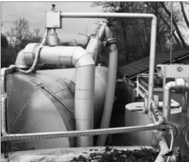
Biogas power plant PHOTO HEIDELBERG ZOO
