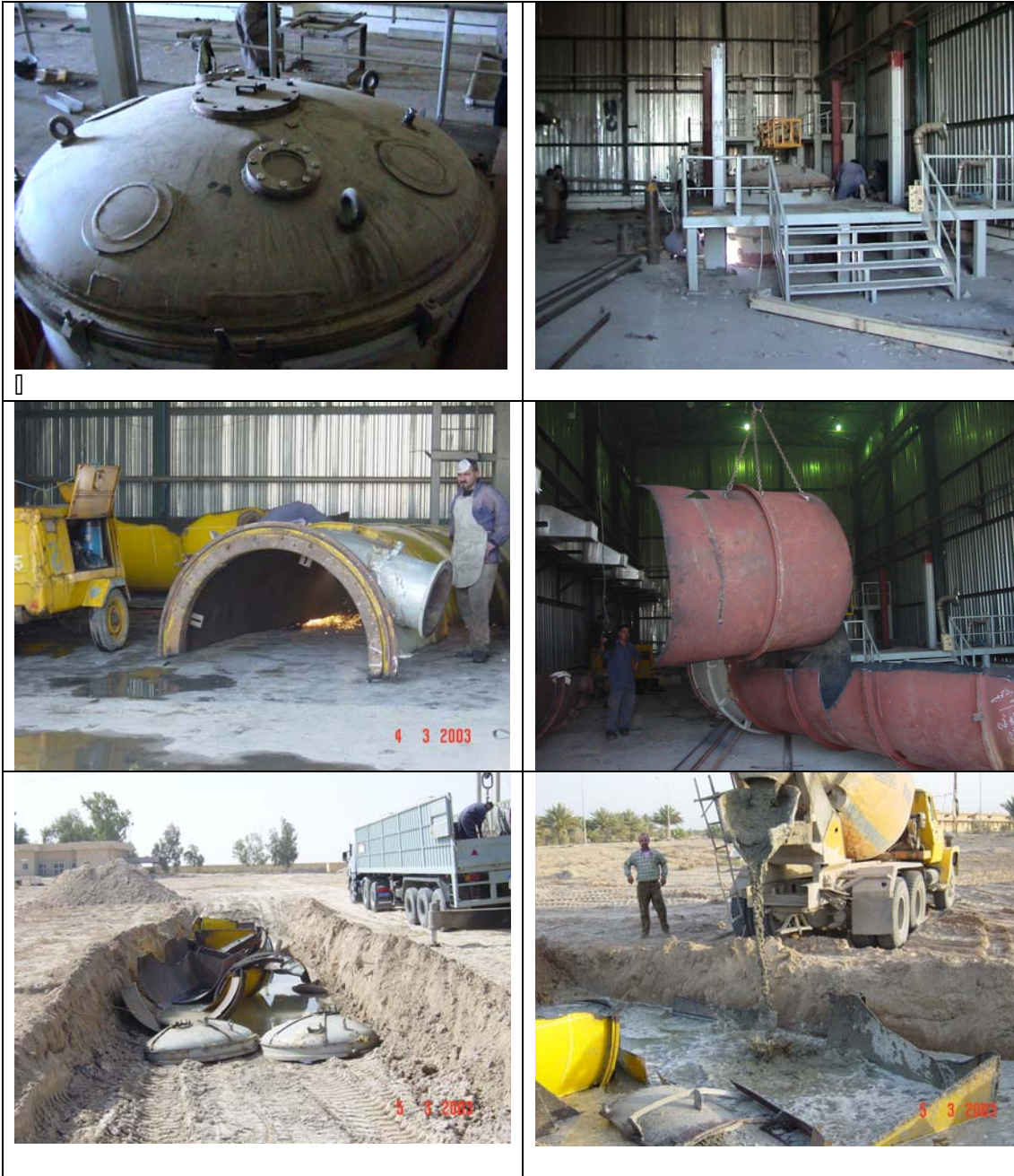
Figure IV.IX.XLV – Destruction of casting chambers
