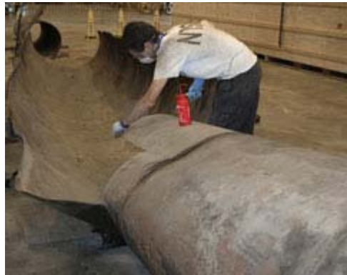
View of ruptured section of pipeline with NTSB investigator cleaning a fracture surface
