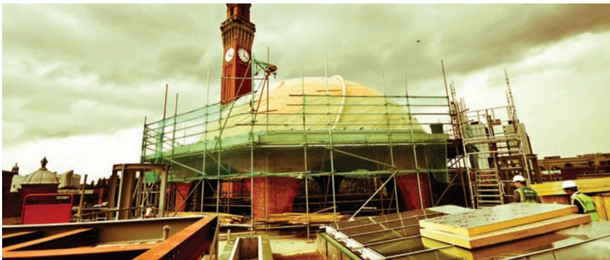
Taking shape: The dome of the new Bramall Music Building, seen in July 2011
