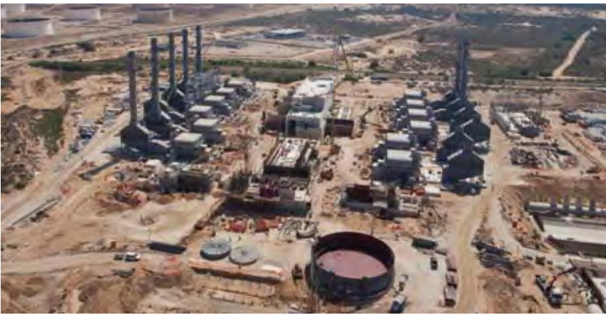
Dorad power plant.
