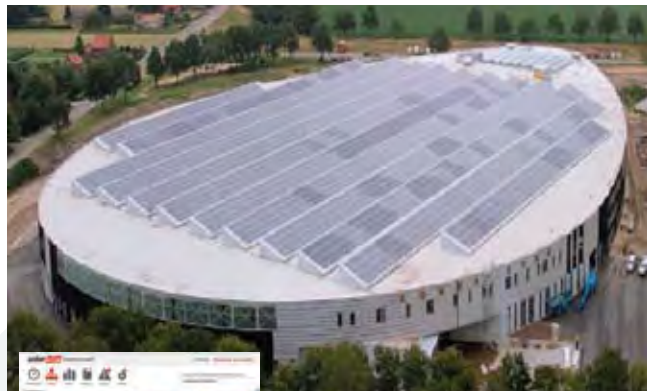
Figure 1: Screenshot from the SolarEdge Monitoring Portal -- Physical layout of a portion of a 1.63 MWp installation in the Netherlands. Specific location of each module on the roof is shown with its specific energy level, for fast and easy troubleshooting and increased system production.
