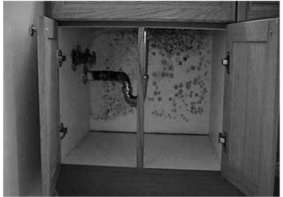
A leaky faucet is the likely cause of the mold growing on the back wall of this cabinet.
