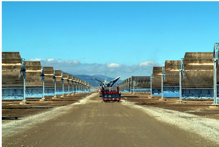
Figure 36. Andasol 1 plant, Solar Millenium, Spain.
