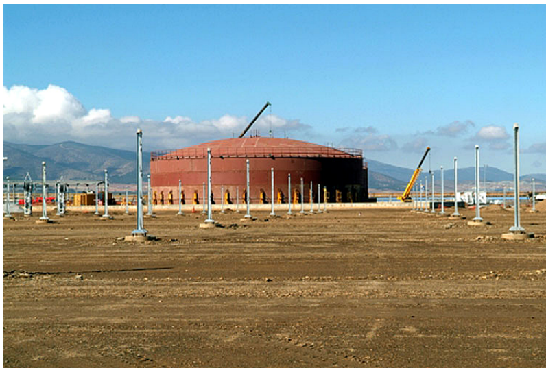
Figure 11. Molten Salt Thermal Energy Storage Tank for electrical power generation, Andasol 1 plant, Spain. Source: Solar Millenium.
