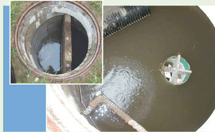
The V2B1's first chamber [right] uses a hydraulic vortex to settle out particles, and then allows clarified water to exit through a central drain into the second chamber [left], where a baffle traps oil and organic debris.
