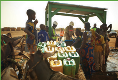
Local residents watch on as Essakane employees install a solar water pump in a neighbouring village.
