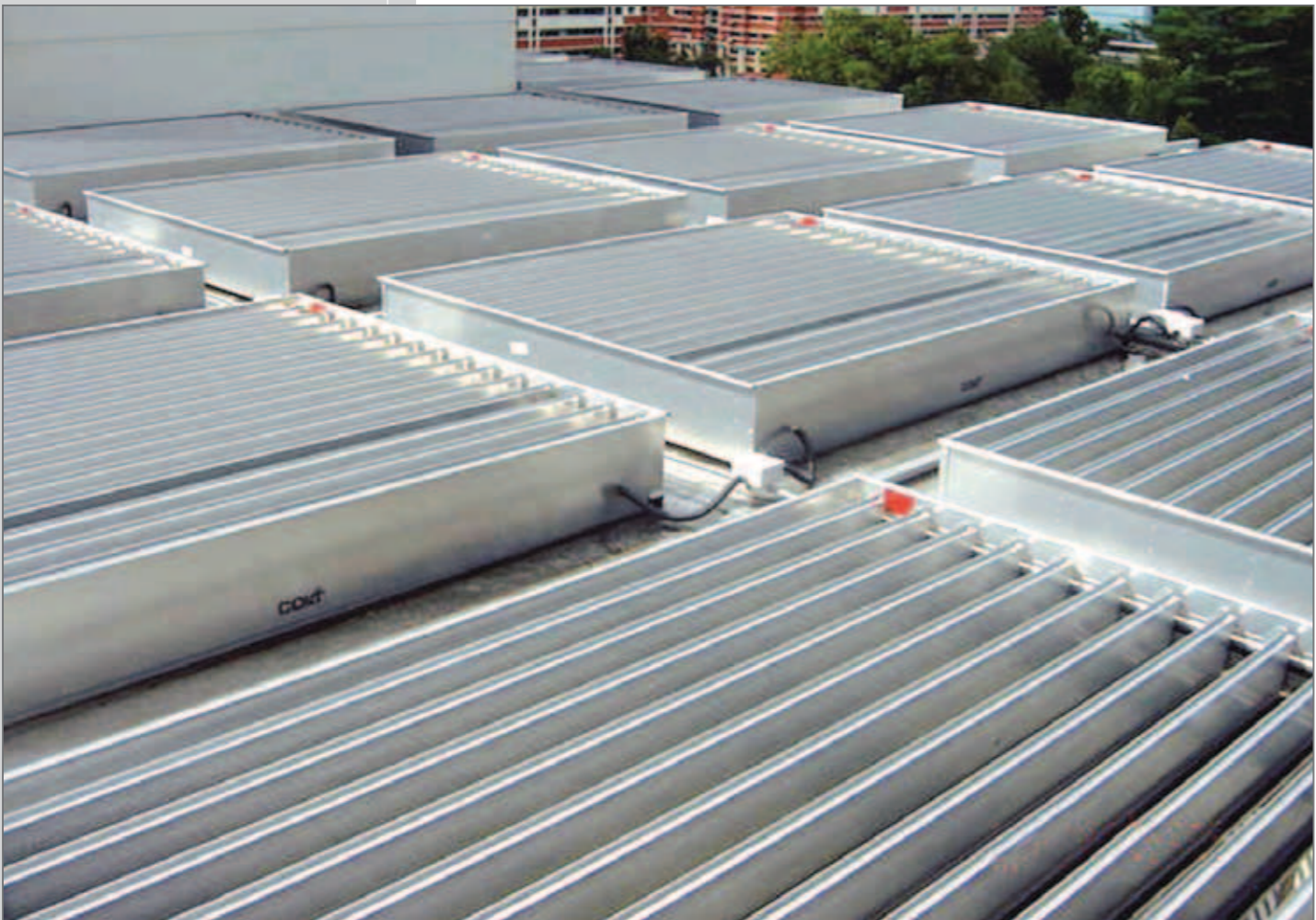
Colt Singapore Singapore Leprosy Relief Association (Silra) Home, Singapore Colt products: EuroCO natural smoke ventilators
