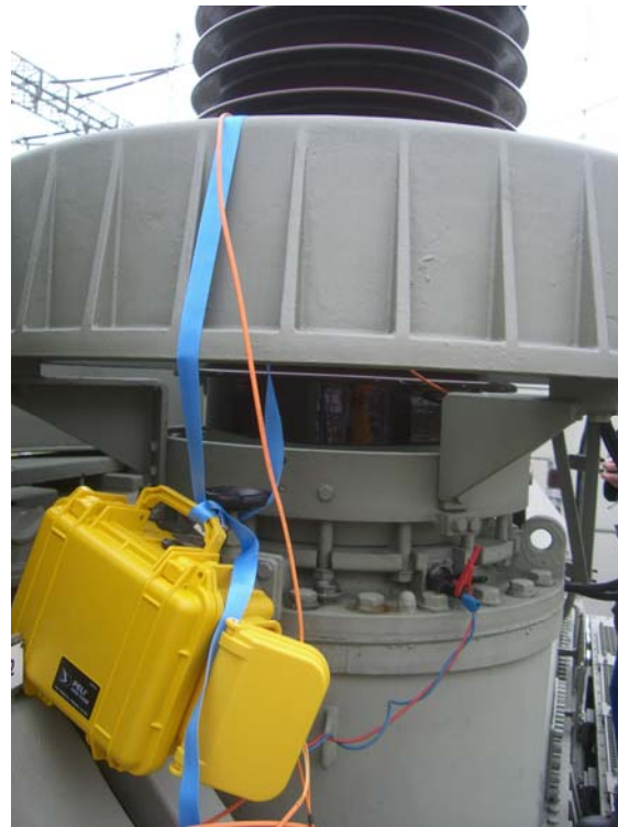
Figure 5 - Connection of the PD system (inside yellow outdoor case) to the measuring tab (420kV bushing).
