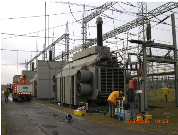
Figure 4 - PD testing of a 333MVA single-phase auto-transformer.
