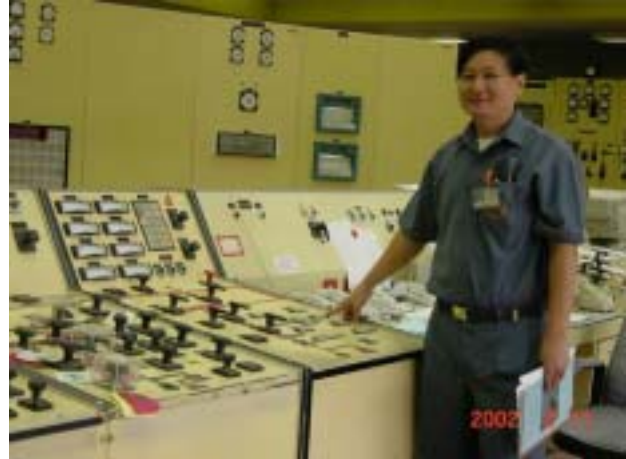
Site Photo : Control Board of Unit 4
