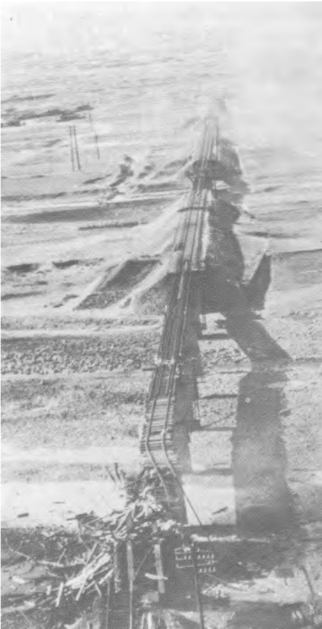
Damaged enemy rail bridge.
