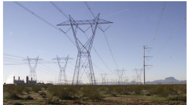
Palo Verde to Pinal West 500 kV Line Salt River Project, Tucson Electric Power Company, Southwest Transmission Cooperative Inc. and Electrical Districts 2, 3 & 4
