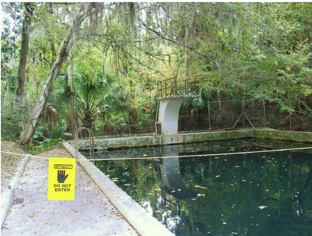
FIGURE 10. VIEW OF GLEN SPRINGS POOL DIVING PLATFORM, FACING SW. (PHOTO BY A. GROSSMAN, 11/22/2010)
