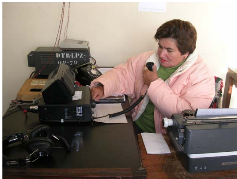
Figure V.1 : Servicio Nacional de Telecomunicaciones Rurales (SENATER), HF radio station in Potosi, Bolivia
