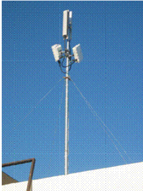
Figure Anx.3.25: Typical WiMAX installation, with two base stations linked to two 60 degree sectored WiMAX antennas
