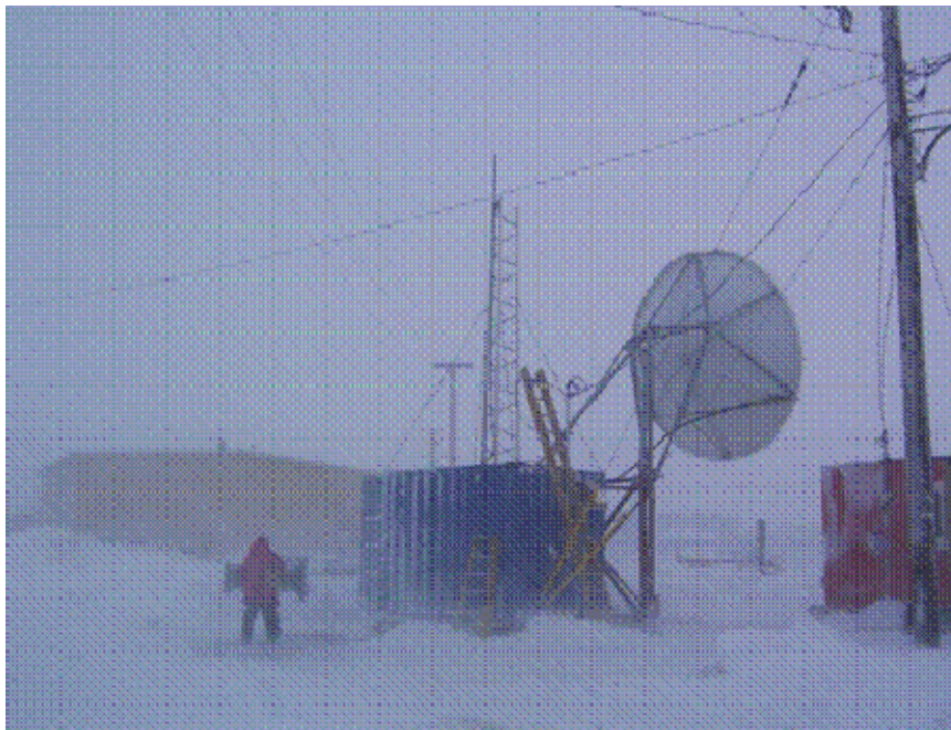
Figure Anx.3.18: QINIQ Network: Installation of 4.5 m antenna, communications shelter and wireless tower at Gjoa Haven, Nunavut, at 68^{\circ} North
