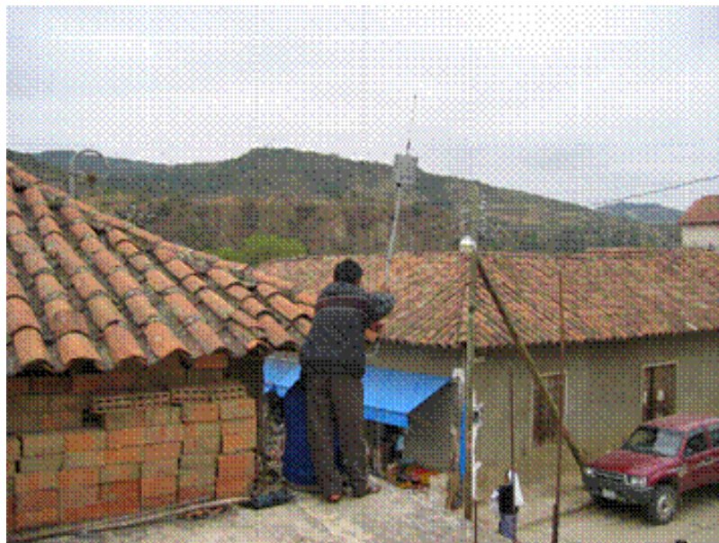
Figure Anx.3.5: Installation of a mesh box at the telecenter, Sopachuy (The omni-directional antenna is located on top of the mesh box)
