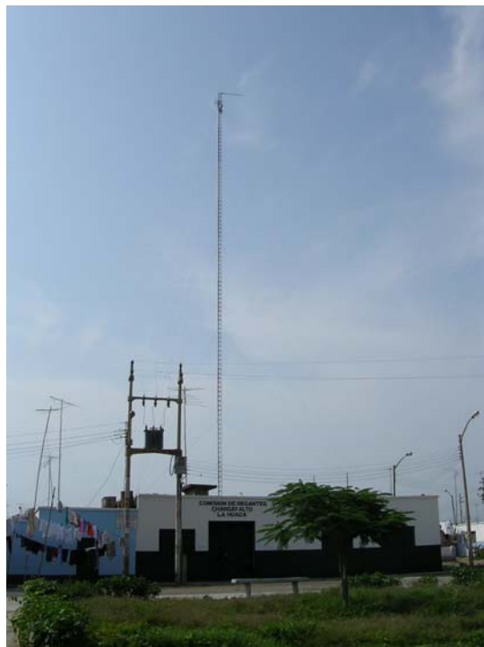
Figure VII.5: Tower and Yagi Directional Antenna of the Chancay–Huaral WiFi backbone network, at the farmers' cooperative in La Huaca, Peru
