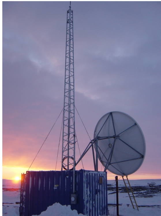
Figure VII.4: QINIQ Network: 4.5 m. VSAT, Base Station Antenna Tower and shelter at Chesterfield, Nunavut, Canada
