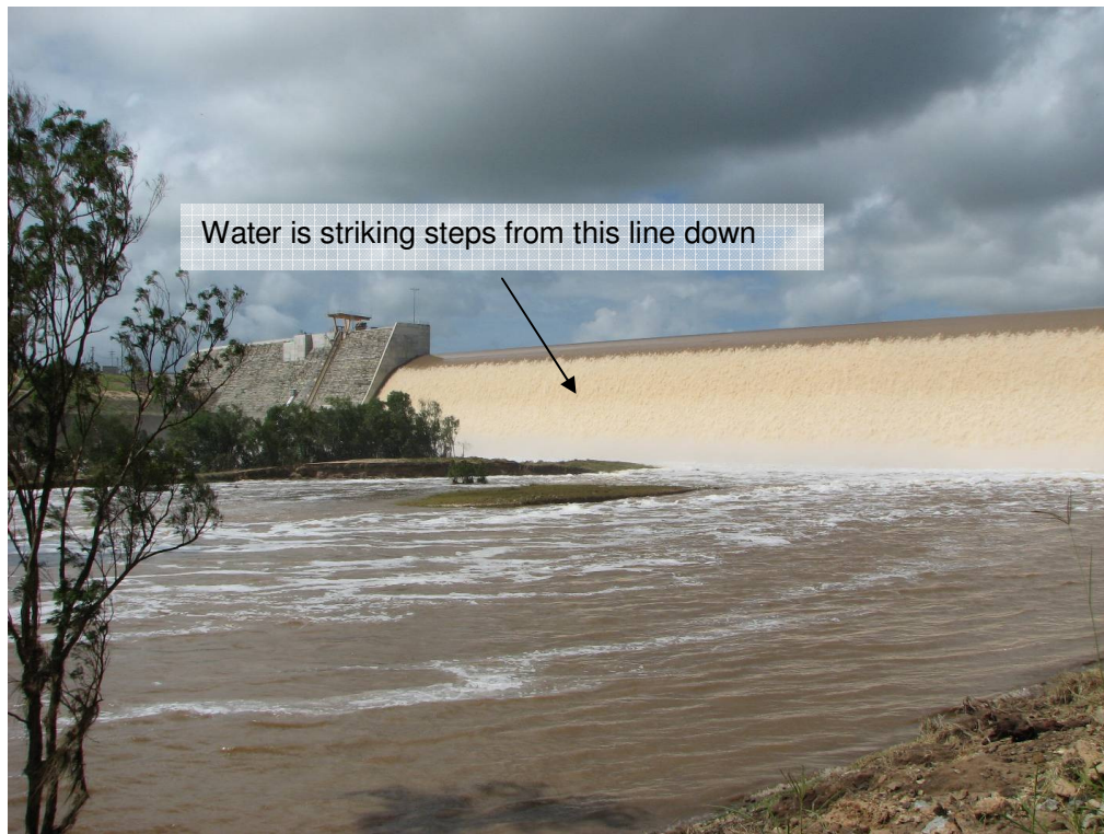
Figure 35 Flows over Paradise Dam at 10 am on the 10th March 2010 at approximately 1.03 m above full supply.
