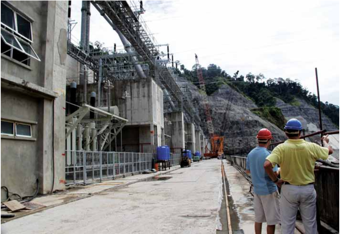
Figure 2: Dr. Sovacool views the powerhouse, spillway and transformer at the nearly-completed 2,400 MW Bakun Hydroelectric Dam
