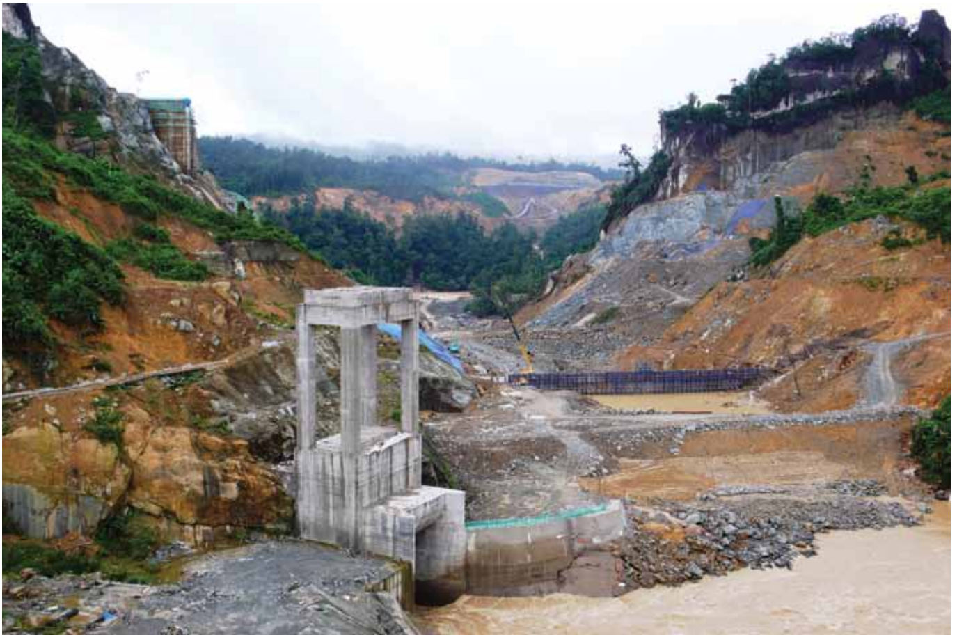
Figure 6: The rock concrete face and powerhouse (located seven kilometers away) of the 944 MW Murum Dam (under construction), July 2010
