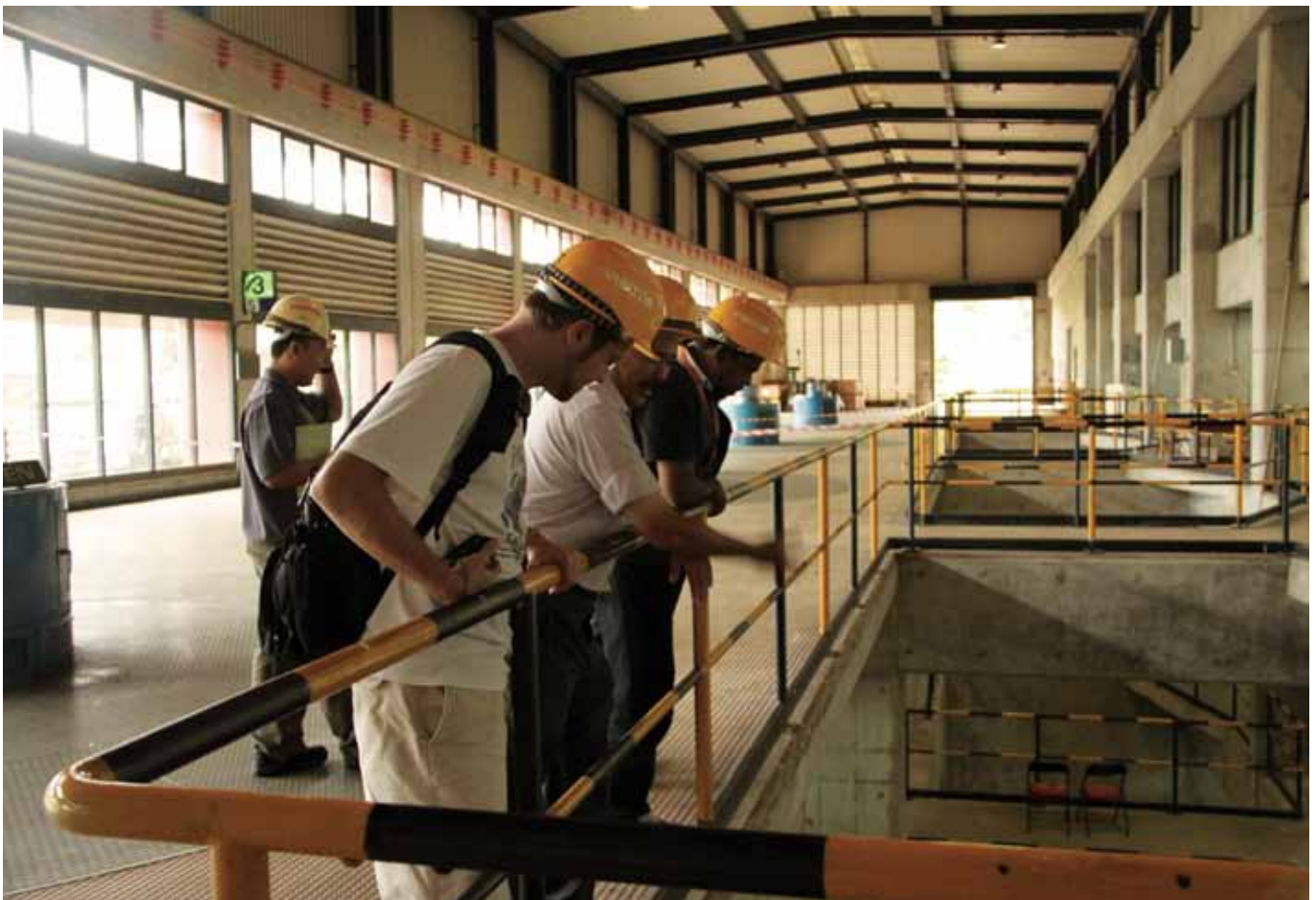
Figure 1: Dr. Sovacool inspects the inside of the 108 MW Batang Ai Hydroelectric Station powerhouse in Sri Aman, Sarawak
