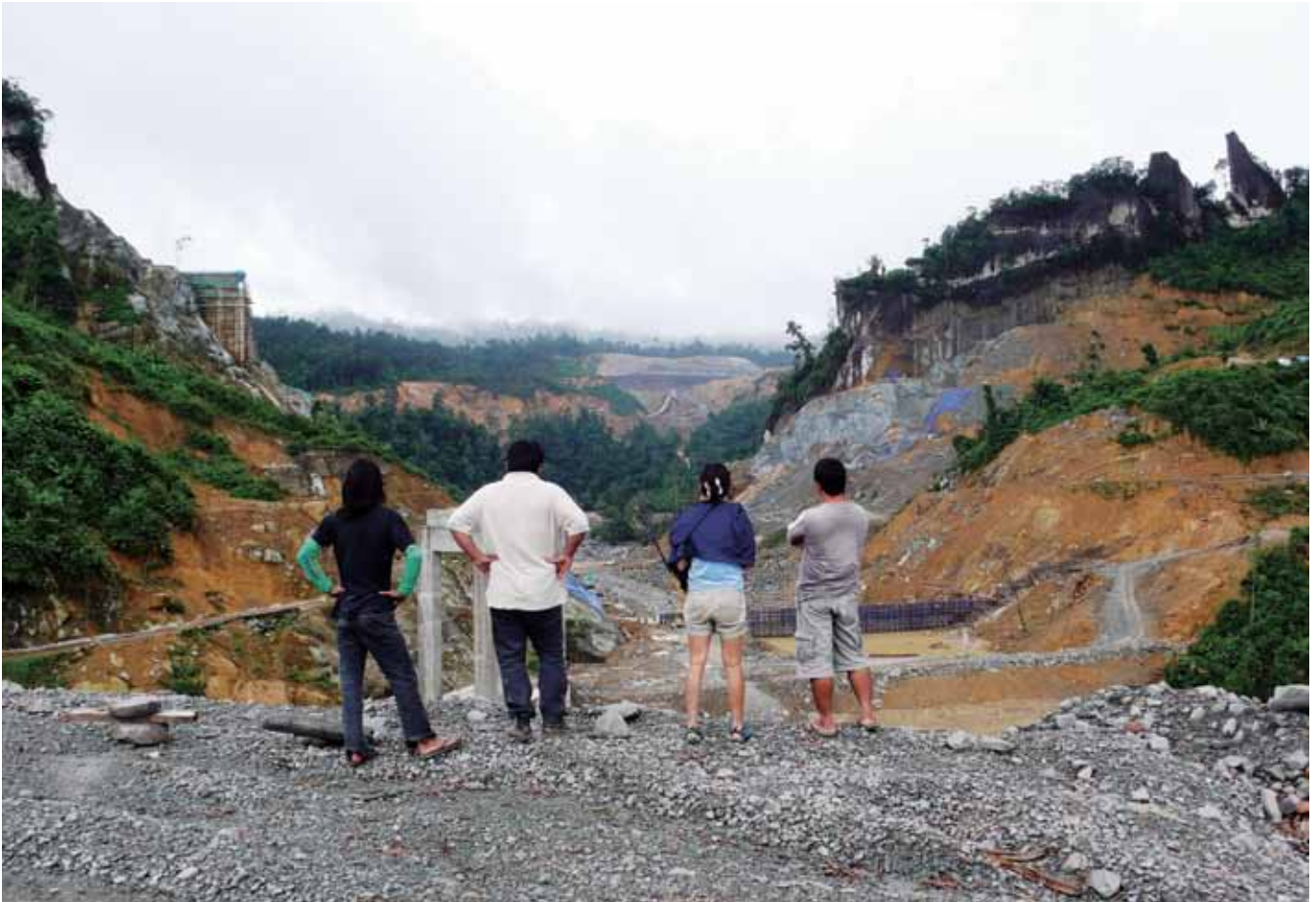
Figure 3: The research team overlooks the under-construction concrete face of the 944 MW Murum Dam in Sarawak
