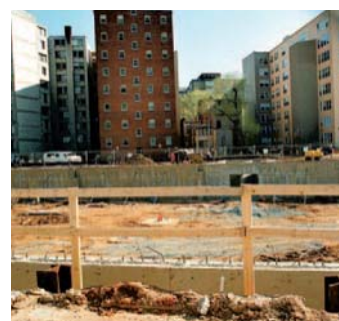
Construction of the P Street Whole Foods, shown in progress in 2000, kick-started 14th Street's transformation.
