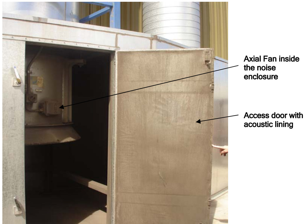
Figure 22: Typical noise enclosure for extraction fans, featuring heavy noise insulating foam sandwiched between perforated metal on the inside and a solid steel outer skin.
