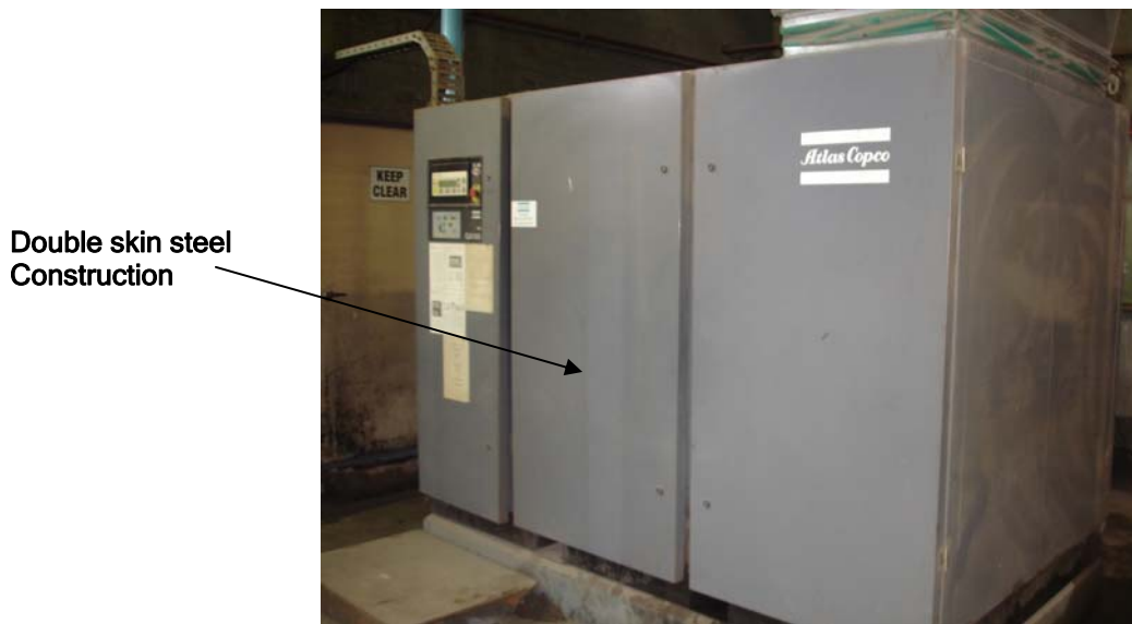
Figure 21: Typical Noise Enclosure to be used for large fans, motors and air compressors
