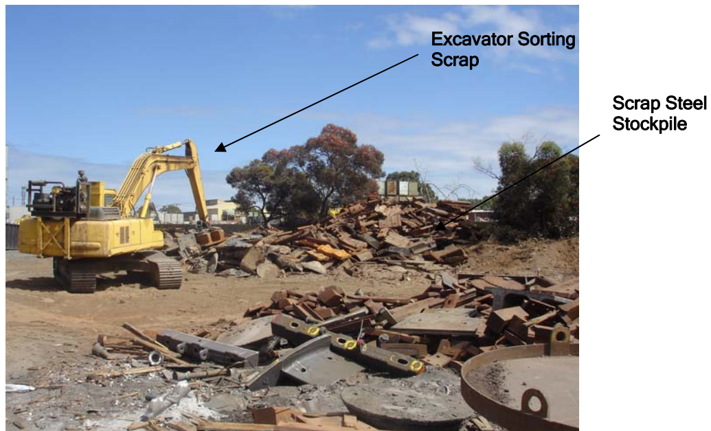
Figure 23: Scrap Handling and sorting using excavator. Currently scrap handling is a source of impact noise. It is proposed that this process is to be relocated to an off site location and only minimum stock of scrap will be held on site.
