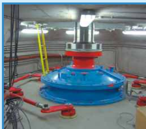
Coupling between Generator and Turbine
