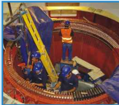
Stator of Power House No. 1
