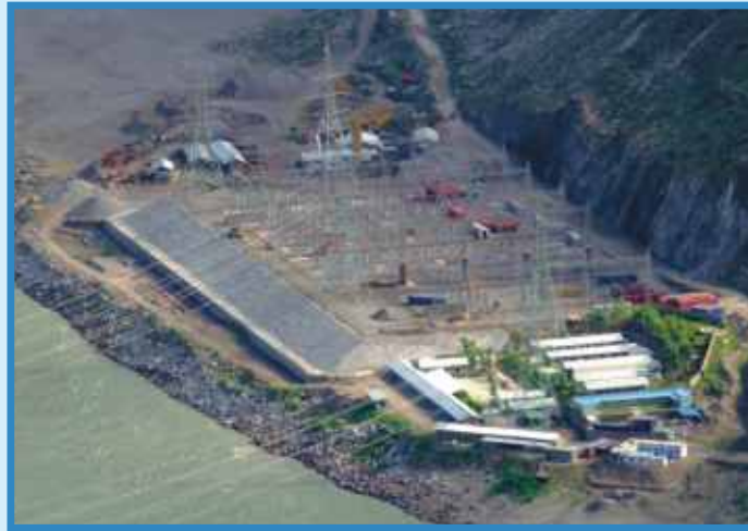
132 kV / 220 kV Allai Switch Yard
