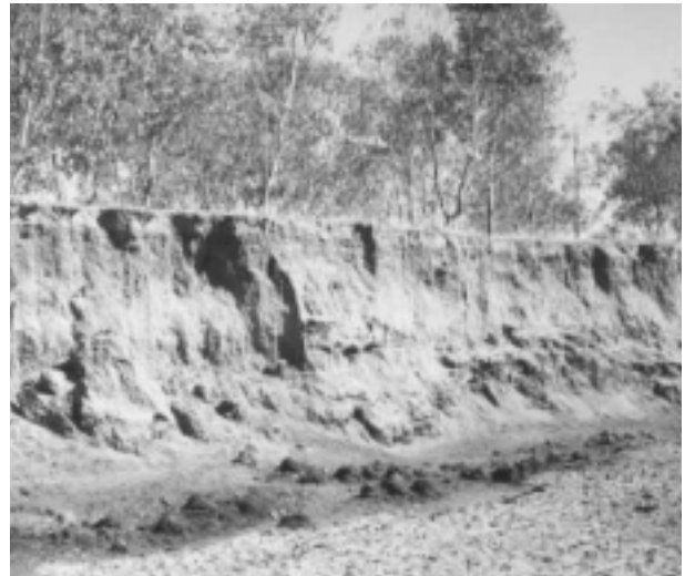
An example of severe bank erosion along Spencers Brook
