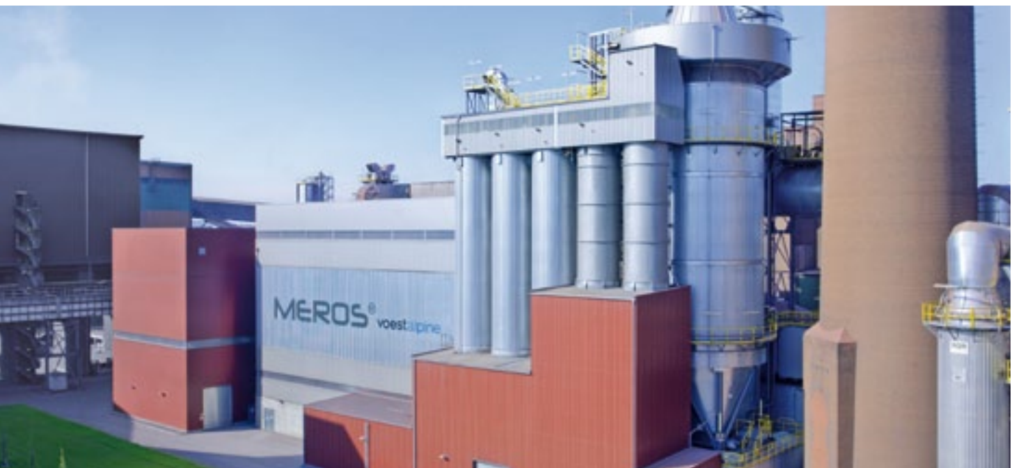
SIMETAL MEROS plant voestalpine Stahl, Linz, Austria
