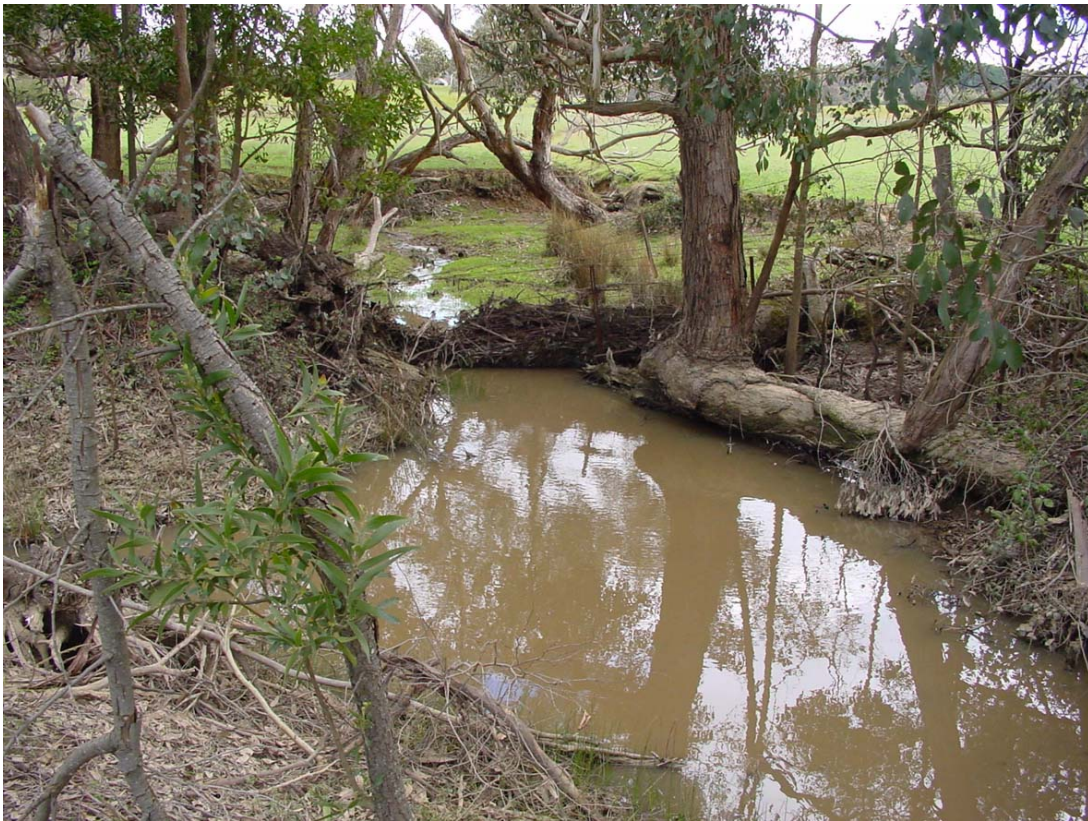
Figure 2 Headcut at 0751958 5822987, looking up the valley onto the intact fill surface. The recently formed channel immediately downstream of the road bridge at this location 1.5 km west of Durham Lead is around 1.5 m deep and several metres wide. This process is generating considerable volumes of sediment, which will be transported downstream. Flow is from left to right. The scarp visible behind the trees is approximately 70 cm high.
