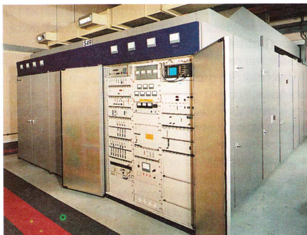
8 One of two 500kW HF sound broadcast transmitters installed at Rampisham, Dorset, for the BBC by GEC-Marconi Communications Ltd.
