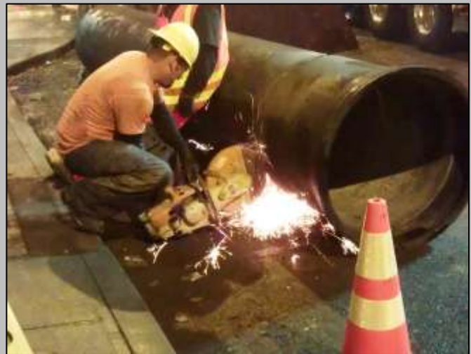
S. Jackson and 7 th – Sunday, October 28 th Preparing 30" water main for installation on 7 th Ave.
