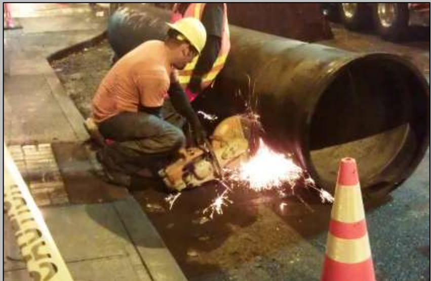
S. Jackson and 7 th – Sunday, October 28 th Preparing 30" water main for installation on 7 th Ave.
