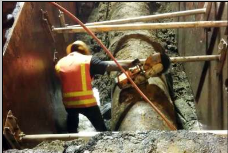
Replacement of a section of this 100 year old 30" water main at 7 th and Jackson is part of the Streetcar's utility work
