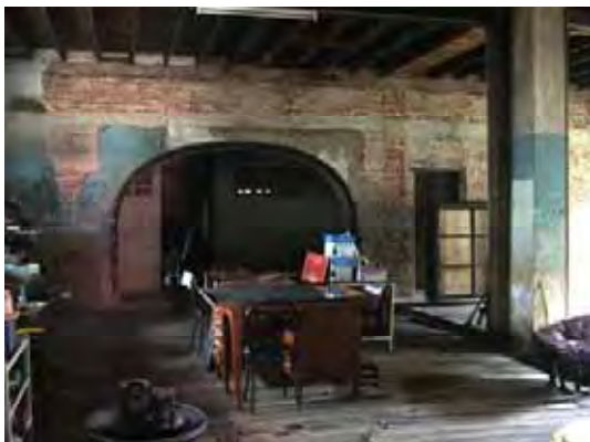
Figure 140: Unfinished renovation part that contains a set of old office desk.
