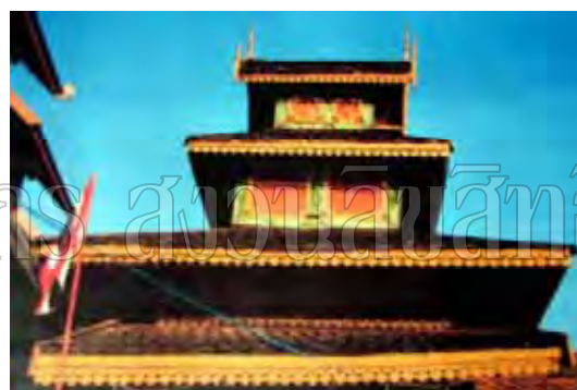
Figure 208: Condition of the tiered roof over staircase before restoration by Fine Arts Department.
