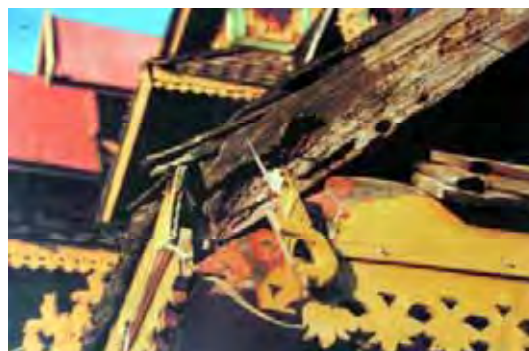
Figure 210: Decayed wood before restoration by Fine Arts Department. (Source: Fine Arts Department, 07.07.2009)
