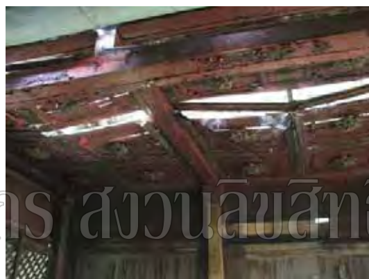
Figure 226: Condition of the ceiling. ( Photograph: 07.11.2008 )
