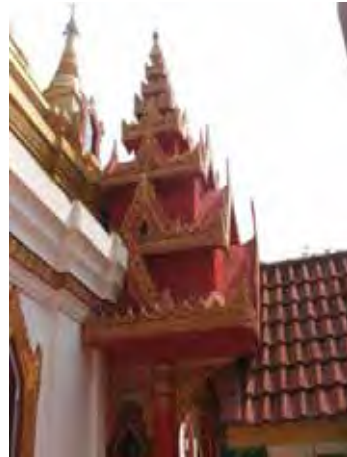
Figure 183: Condition of pyathat porch. ( Photograph: 19.02.2009 )
