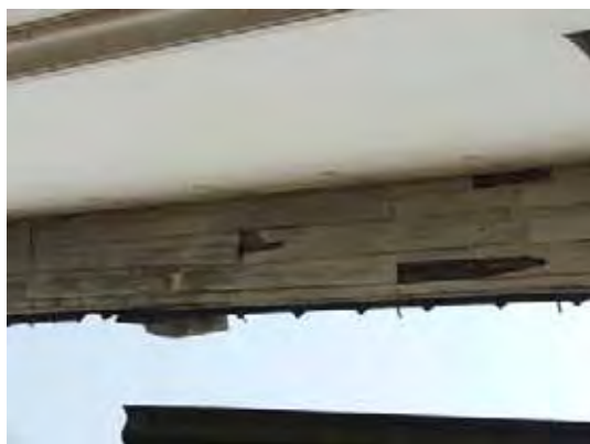
Figure 238: Decayed wood beneath eave wings.
