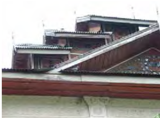
Figure 195: Condition of the upper part of monastery.
