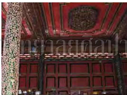
Figure 176: Condition of interior of the monastery. (Photograph: 17.11.2008)
