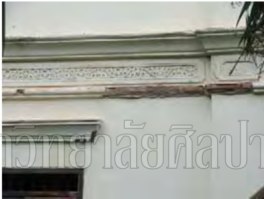
Figure 199: Ruined stucco reveals the structure.
