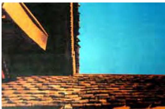
Figure 209: Condition of the traditional clay roof tiles before restoration by Fine Arts Department. (Source: Fine Arts Department, 07.07.2009)
