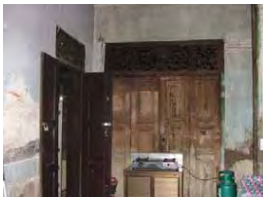
Figure 240: Efflorescent and fragment on the wall.
