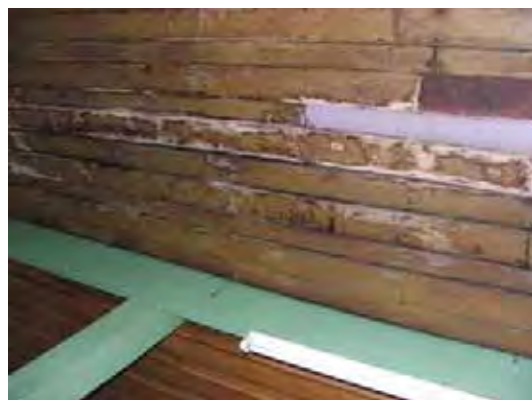
Figure 241: Leakage left its trace on wood ceiling.
