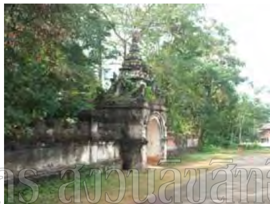
Figure 220: Condition of the second gatehouse with lichen and weeds growing on top.
