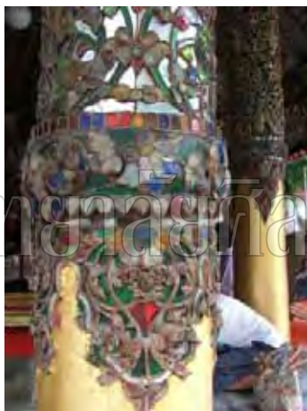
Figure 164: Missing colored glass.
