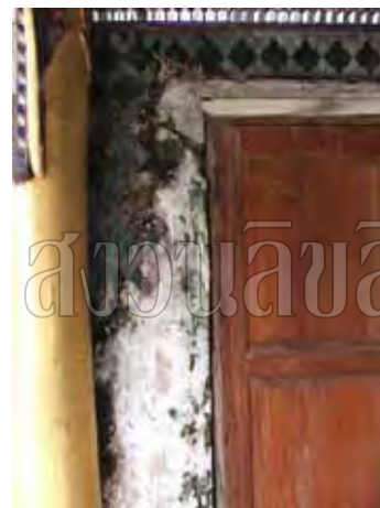
Figure 165: Efflorescence and lichen on the wall.
