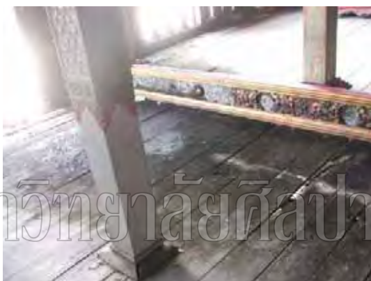
Figure 225: Condition of the floorboard. ( Photograph: 07.11.2008 )
