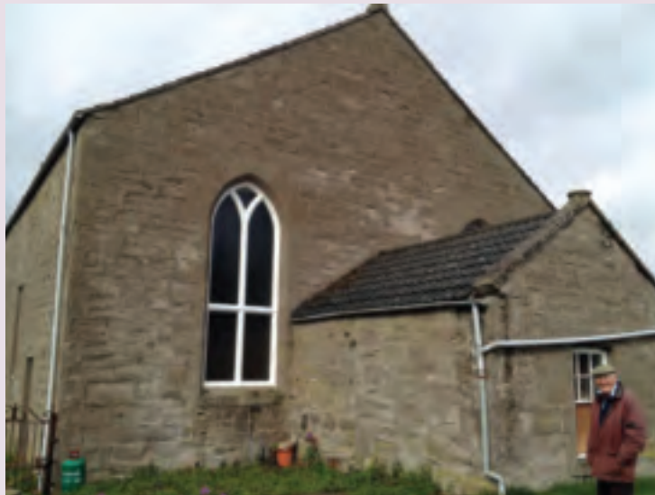
One of the replacement windows at Balbeggie and Collace United Free Church of Scotland
