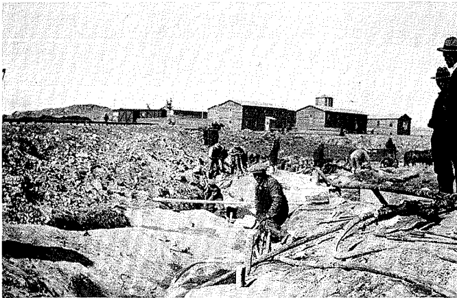
Drilling in preparation for blasting. Bunkhouses were built to house the construction workers. (H. Ennis 1929)
