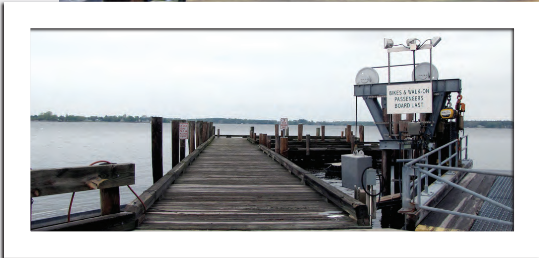
The Town of Oxford's Timber Dock was re-configured, expanded and rebuilt to accommodate larger, recreational transient boats. The former dock had been deteriorating.
