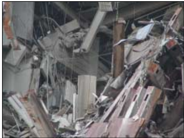
Figure 3.26. Exterior and interior damage to the Banker's Trust Building
