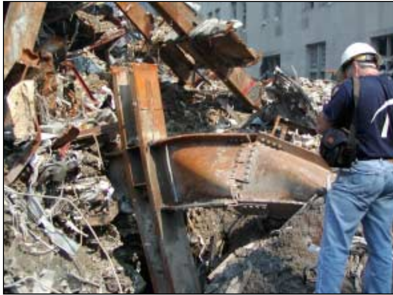
Figure 3.14 Distorted segments of beam stubs welded to the columns
