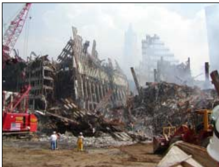
Figure 3.5. Portions of the perimeter tubes of WTC 1 and 2 remained standing in the debris pile (as of September 21, 2001)
