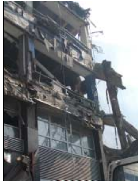
Figure 3.16 Damage to the west face of a building at 30 West Broadway due to impact from the collapse of WTC 7
