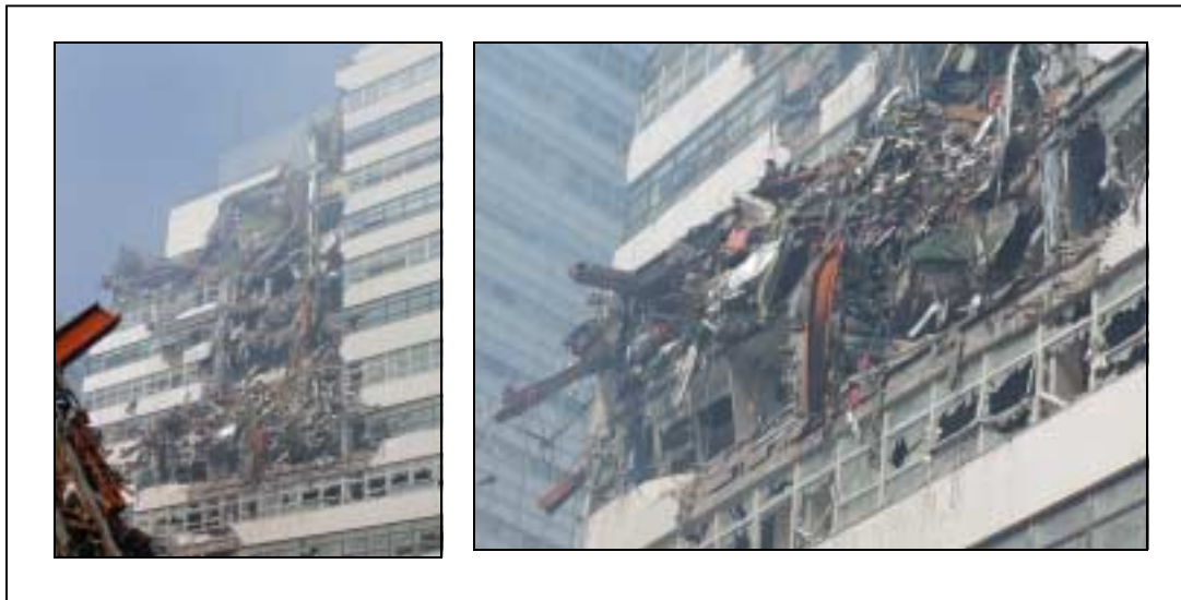
Figure 3.15. Damage to the south face of a building at 30 West Broadway due to impact from the collapse of WTC 7
