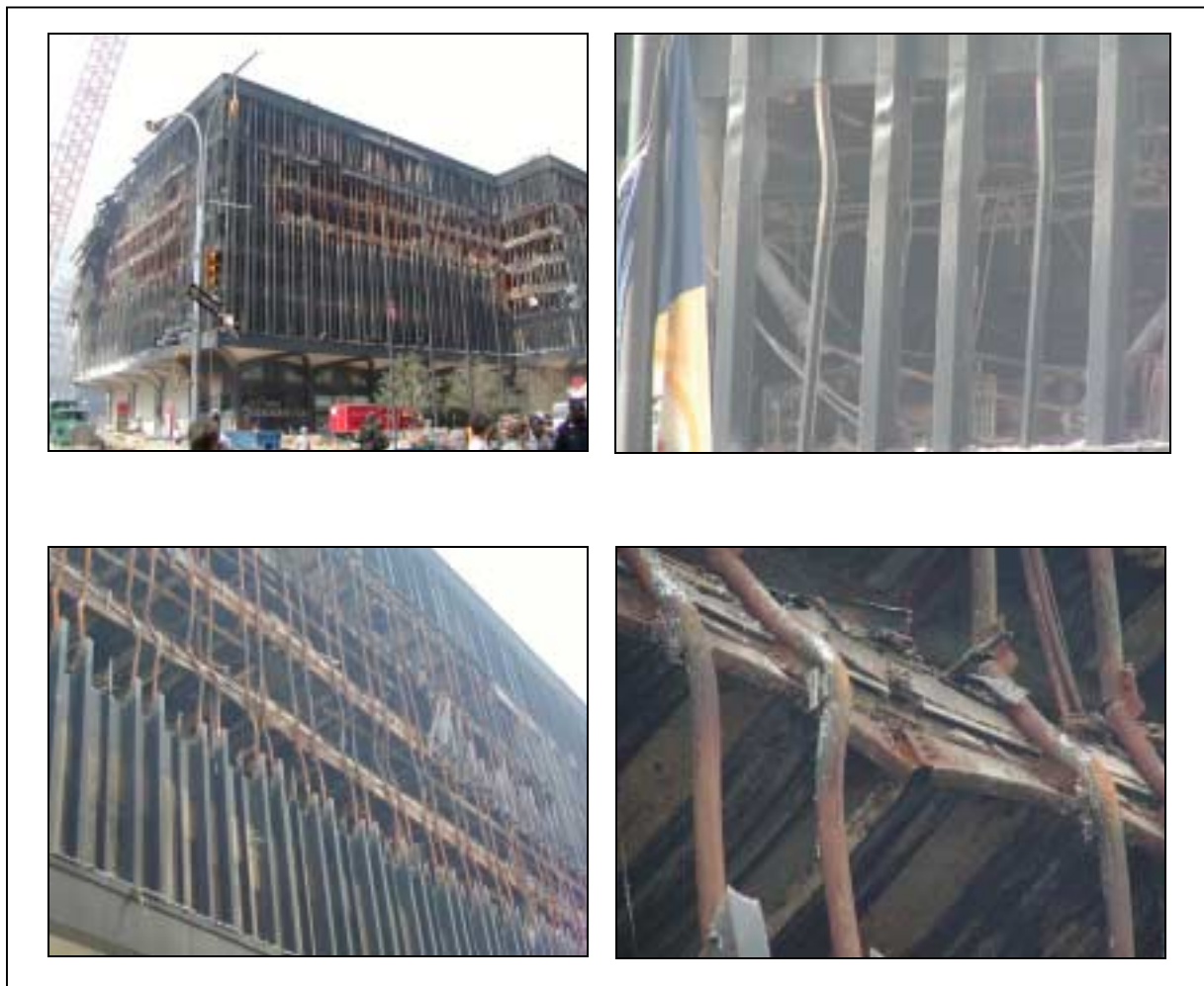
Figure 3.10. Fire related damage to WTC 5
