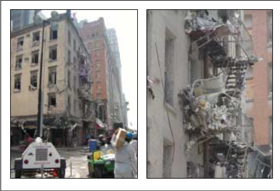
Figure 3.29. Debris in the emergency stairs of a small building near Ground Zero
