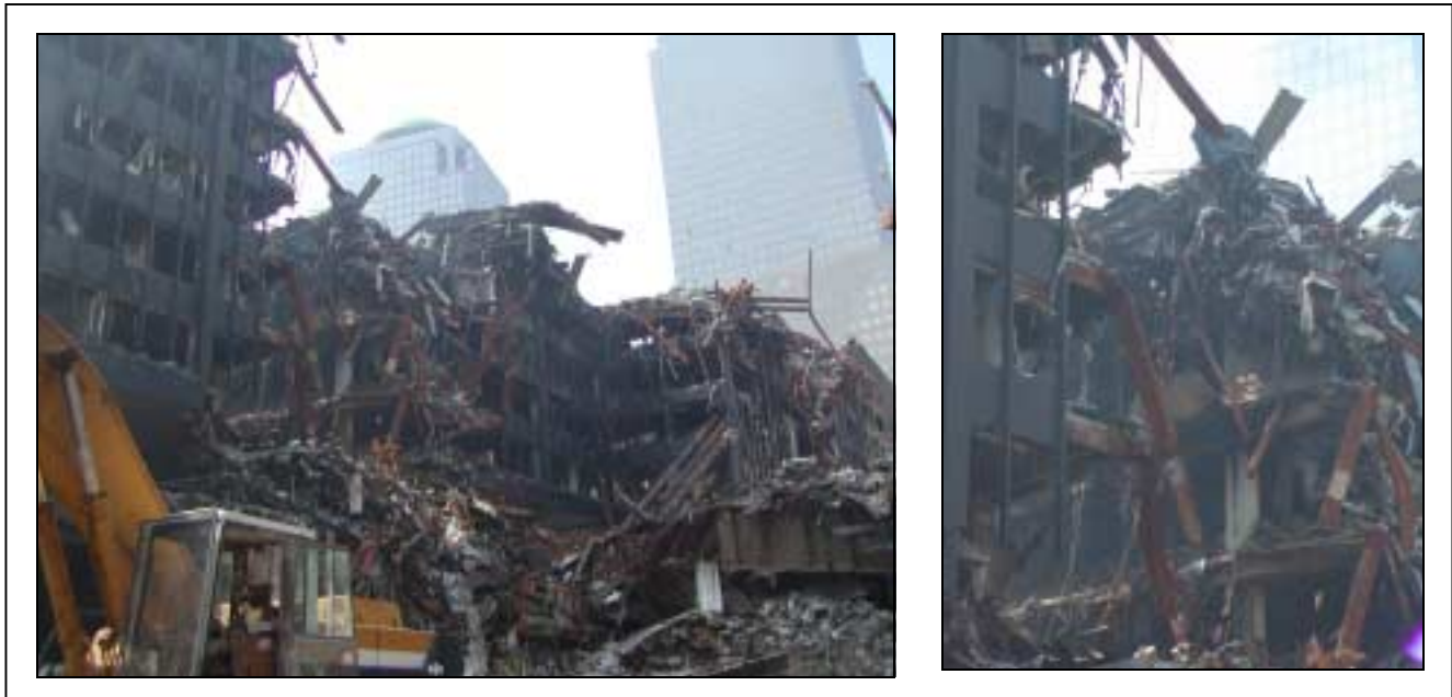
Figure 3.11. Impact and fire-related damage to WTC 6
