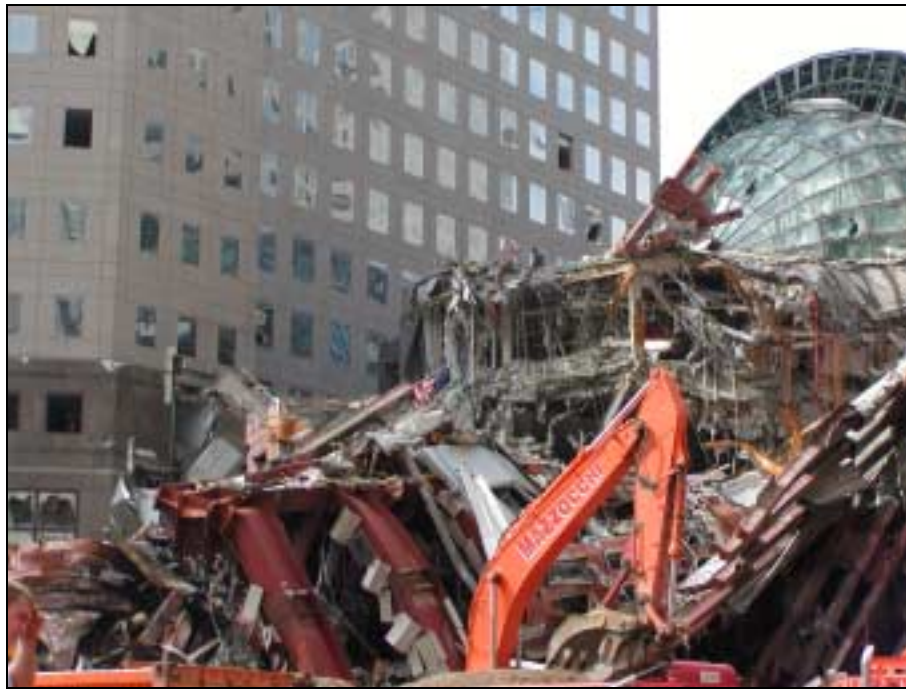
Figure 3.21. Severe damage to the east side of the Winter Garden
