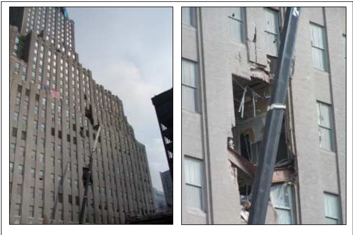
Figure 3.19. Minor damage to south façade of the Verizon building
