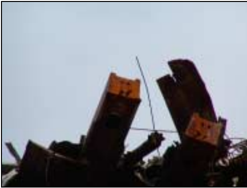
Figure 3.7. Typical four-bolt column splices and access holes on the side of hollow rectangular columns
