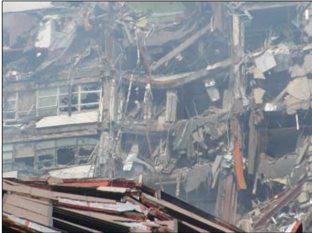
Figure 3.17. Beams in the building at 30 West Broadway were permanently distorted by the impact of falling debris
