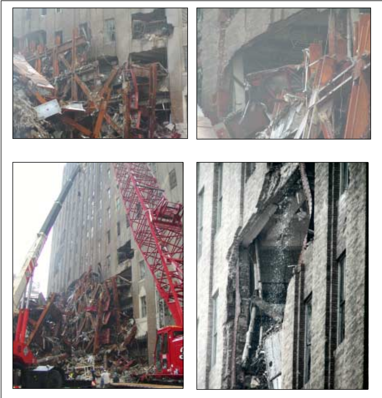
Figure 3.18. Damage to the west façade of the Verizon Building
