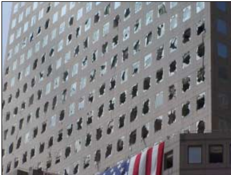
Figure 3.27. Broken windows in 2 World Financial Center
