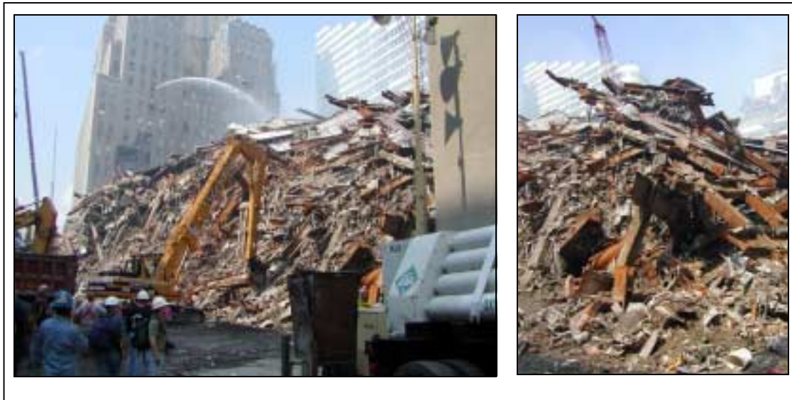
Figure 3.12. WTC 7 collapsed as a consequence of damage and uncontrolled fire
