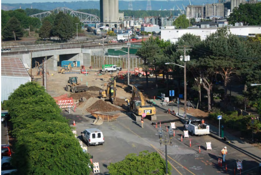
Waterfront Access Construction Project Reconnecting Downtown Vancouver to the vital Columbia River
