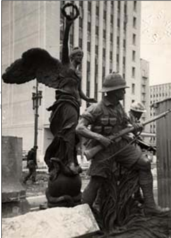
Photograph 3.54: Deconstruction of Cenotaph in 1959 due to Adderley Street widening, National Library of South Africa, Special Collections
