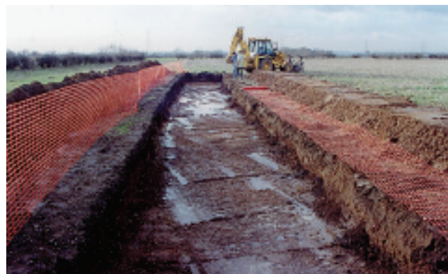
Excavation of an evaluation trench near the Roman town of Crococalana, Brough, Nottinghamshire (photograph: H. Jones)
