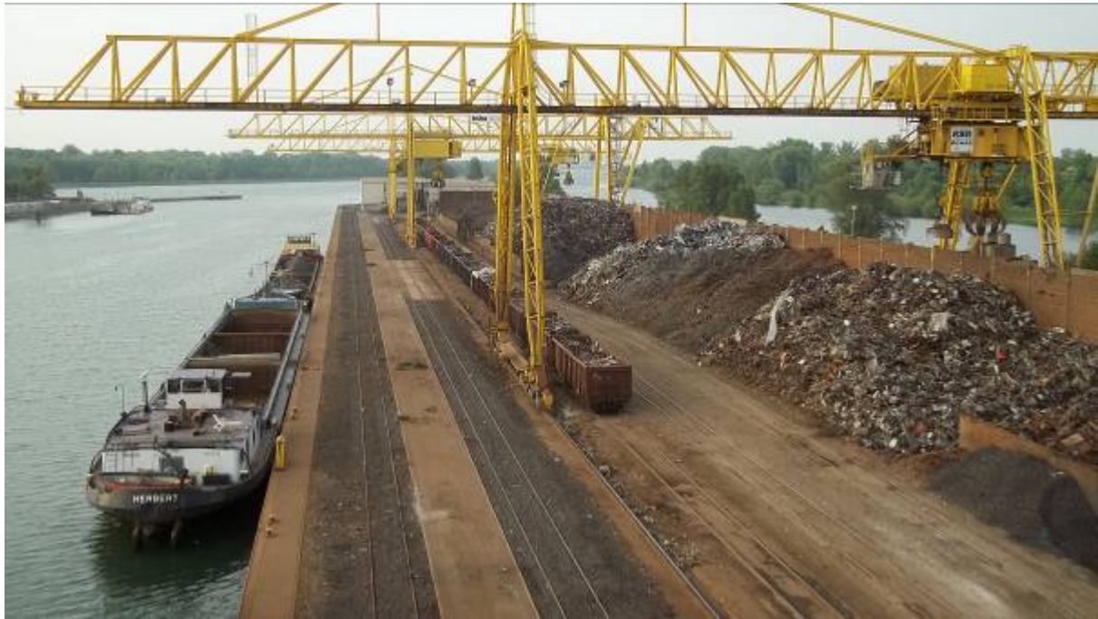
Picture 7: Scrapyard with 3 tracks for scrap ferry, 2 railway tracks and 1 crane rail. Railway wagons ready for unloading
