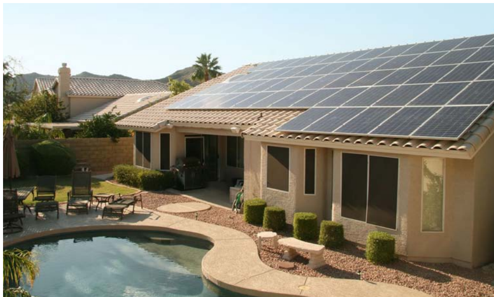
Residential PV Installation in Arizona
