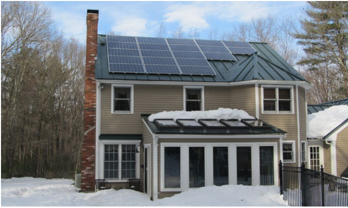
Residential PV Installation in Massachusetts
