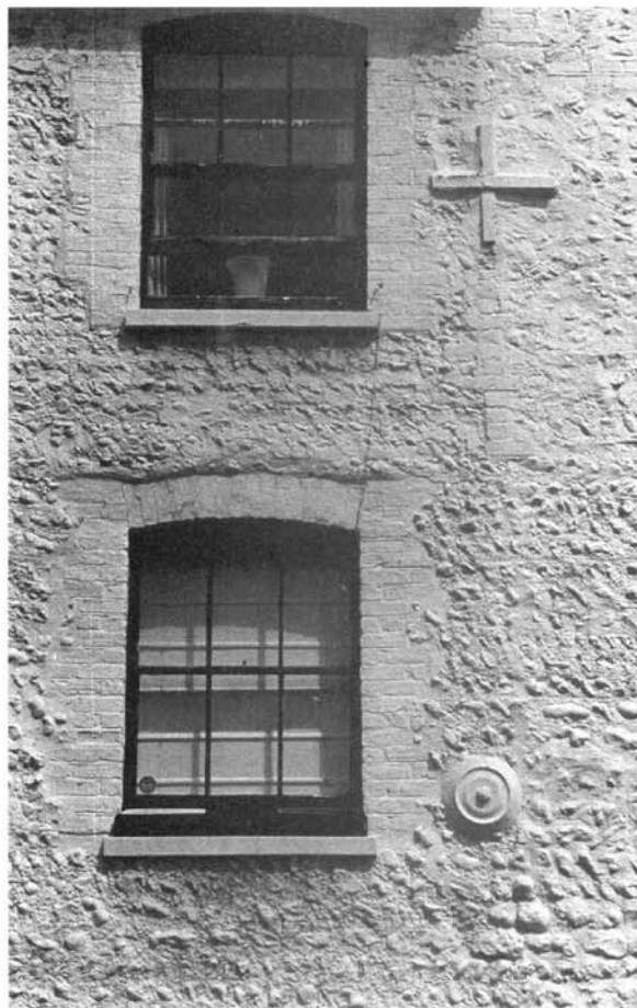
Rear of Kemp Town Place elevation, showing cast iron wall-tie plates
