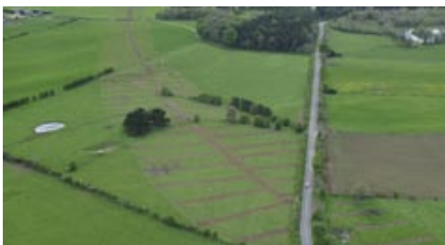
a: Test trenching carried out as part of the archaeological testing of the M7 Portlaoise–Castletown/M8 Portlaoise–Cullahill motorway scheme (Narrowcast, courtesy of the NRA)
