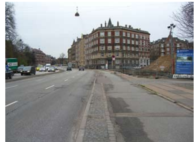
A bridge is currently being constructed which will go over Ågade, a busy main street that connects with H.C. Andersens Boulevard.
