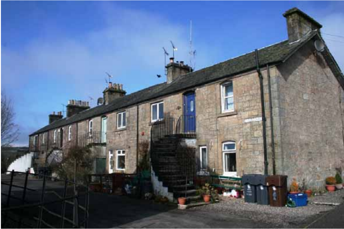
Fig 3: the 'rear' façade of the south-west range of The Square. Properties were designed as flatted houses with attractive curved entrance stairs contrasting with the otherwise regular form of the buildings. Note there has been considerable detrimental change to this block, including inappropriate replacement window types and widening of the original single arched windows.
