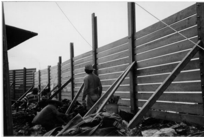
Figure 5 - The contention wall built to protect the station against strong sea waves.
