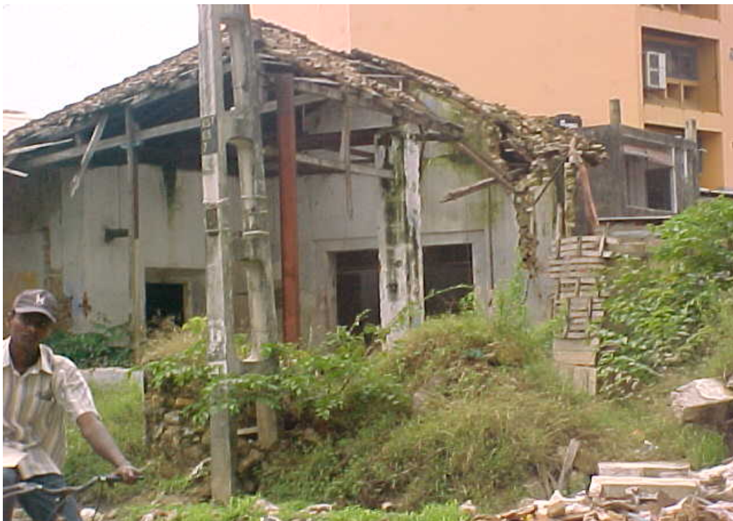
Tsunami affected building at Magalla Note debris not cleared
